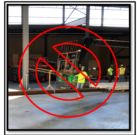
INCORRECT SUSPENDED LOAD
